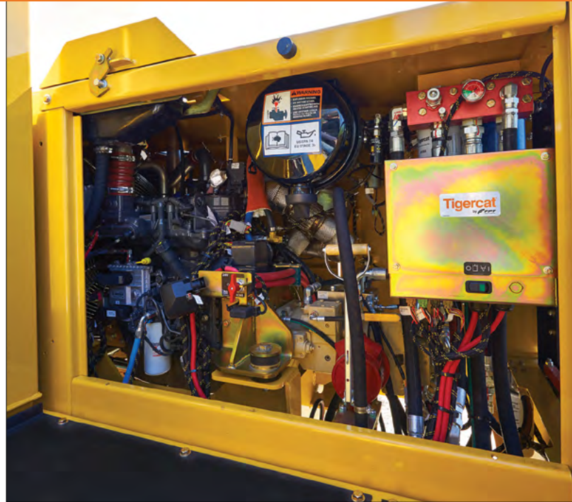
Convenient platform access to the engine and daily service points. The compartment is neat and spacious.
